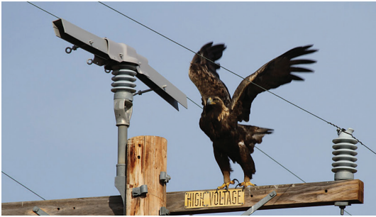
It is estimated that perhaps millions of birds, including Bald and Golden Eagles, owls, and hawks die each year as a result of power line interactions. Photo used with permission © Debi Shearwater
